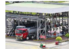
Bulk Filling Gantry
